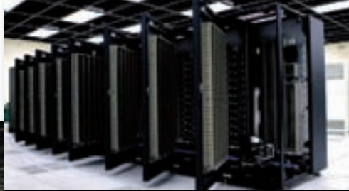
PHOTOS PROVIDED BY OREGON STATE DATA CENTER
